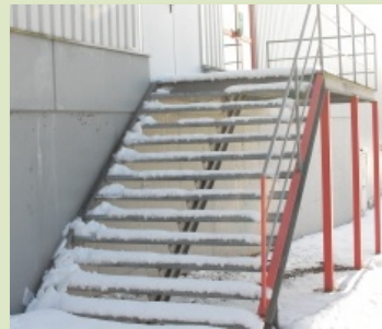
Illustration 32: Iced-over stairs [Source: ikl]
