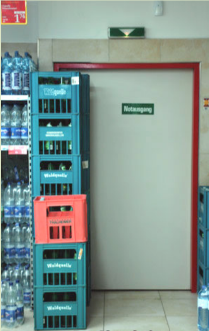
Illustration 30: Blocked emergency exit [Source: ikl]
